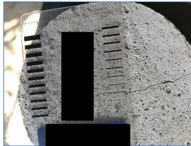
T-④ひび割れ幅0.2mm
